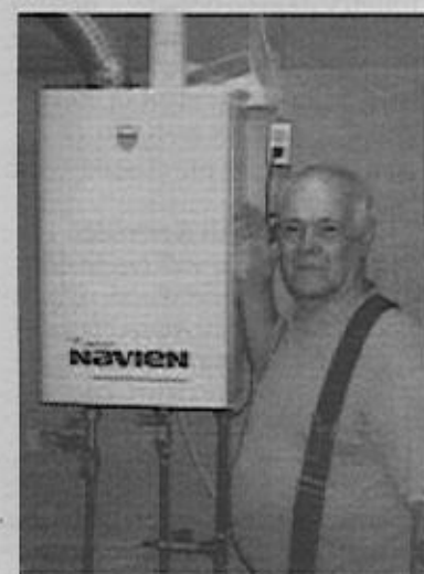
R.:W.: Richard Snyder beside the new on-demand water heater installed in the bath house at Camp DeMolay.
